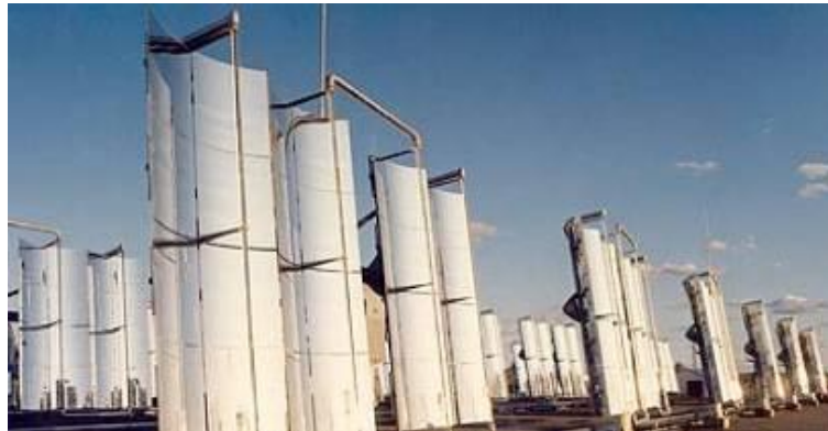
Figure 3-6: Meekatharra Collectors, (WA World of Energy).
